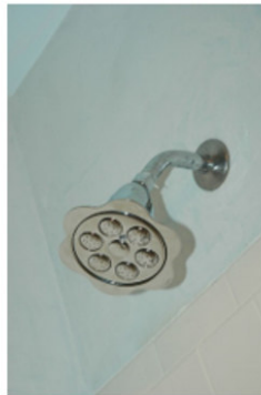
Picture 2: The shower head protrudes from the wall.
